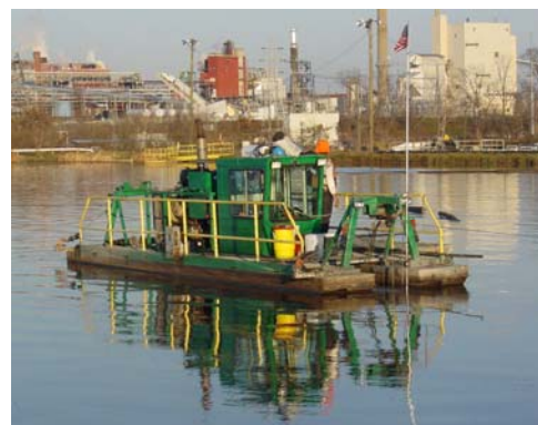
Eagle has extensive experience in dredging to a process. This operation involved dredging a consistent flow of material to a dewatering process 24 hours per day, 7 days per week for approximately 14 months.
