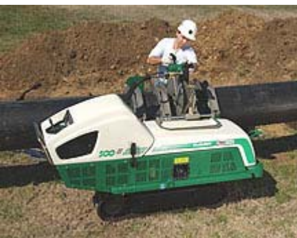
Eagle utilized track mounted fusion machines to increase productivity and allow for safer pipe installation. Eagle has pipe fusion capability from 4" to 20".
