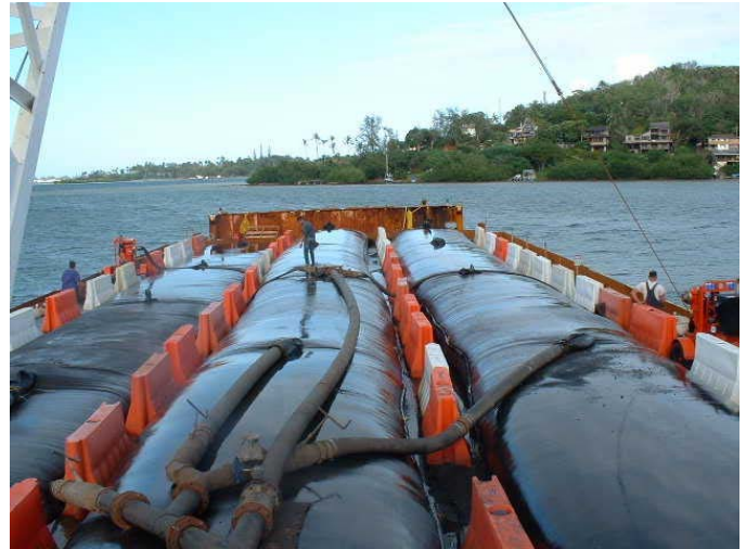
Eagle specializes in more difficult dewatering applications. This project involved the removal of contaminated sediments in Hawaii, the sediments were dewatered using geotubes on a barge. The filtrate was required to be captured and sampled prior to release. The dewatered sediments were off-loaded from the barge for disposal.
