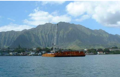
Eagle has extensive experience working outside of the mainland of the US, the above project was recently completed in Hawaii.
