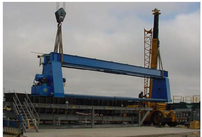
Installation of Eagle's High Pressure Membrane Filter Press at INCO located in Thompson, Manitoba.
